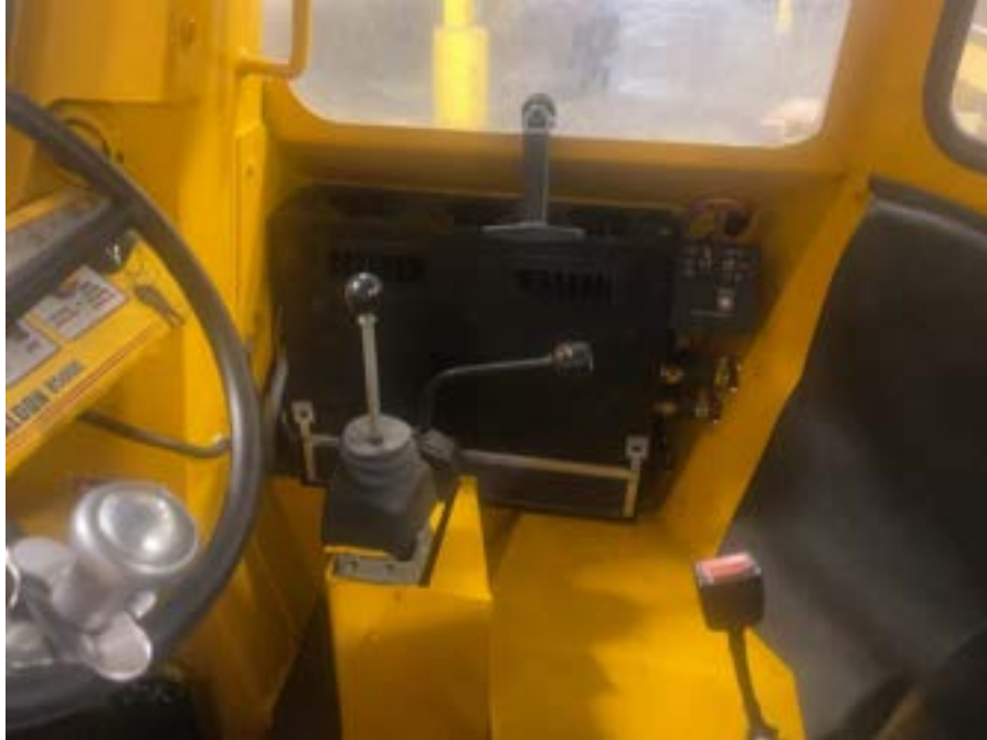
Switches and Controls
